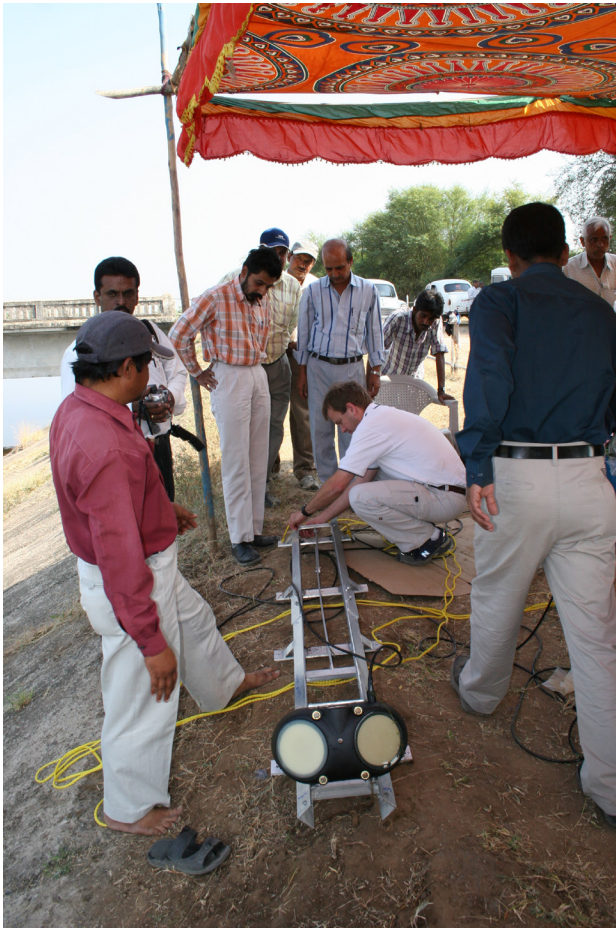
Installation of a Argonaut-SL500 (“side-looking”) into the Narmada canal.
