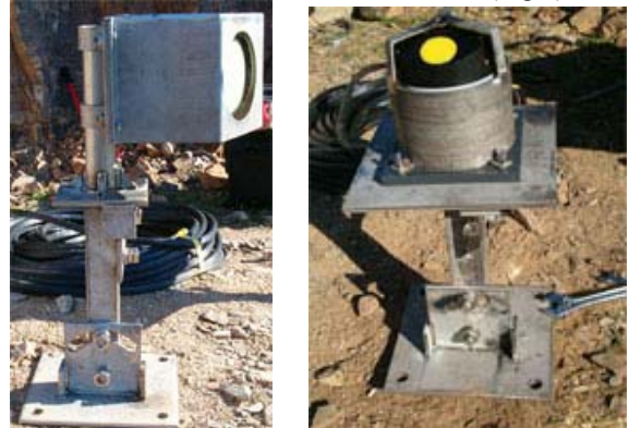
Fig 5. Steel structures which fix the sensors to the concrete cubes (SL left and XR right).
